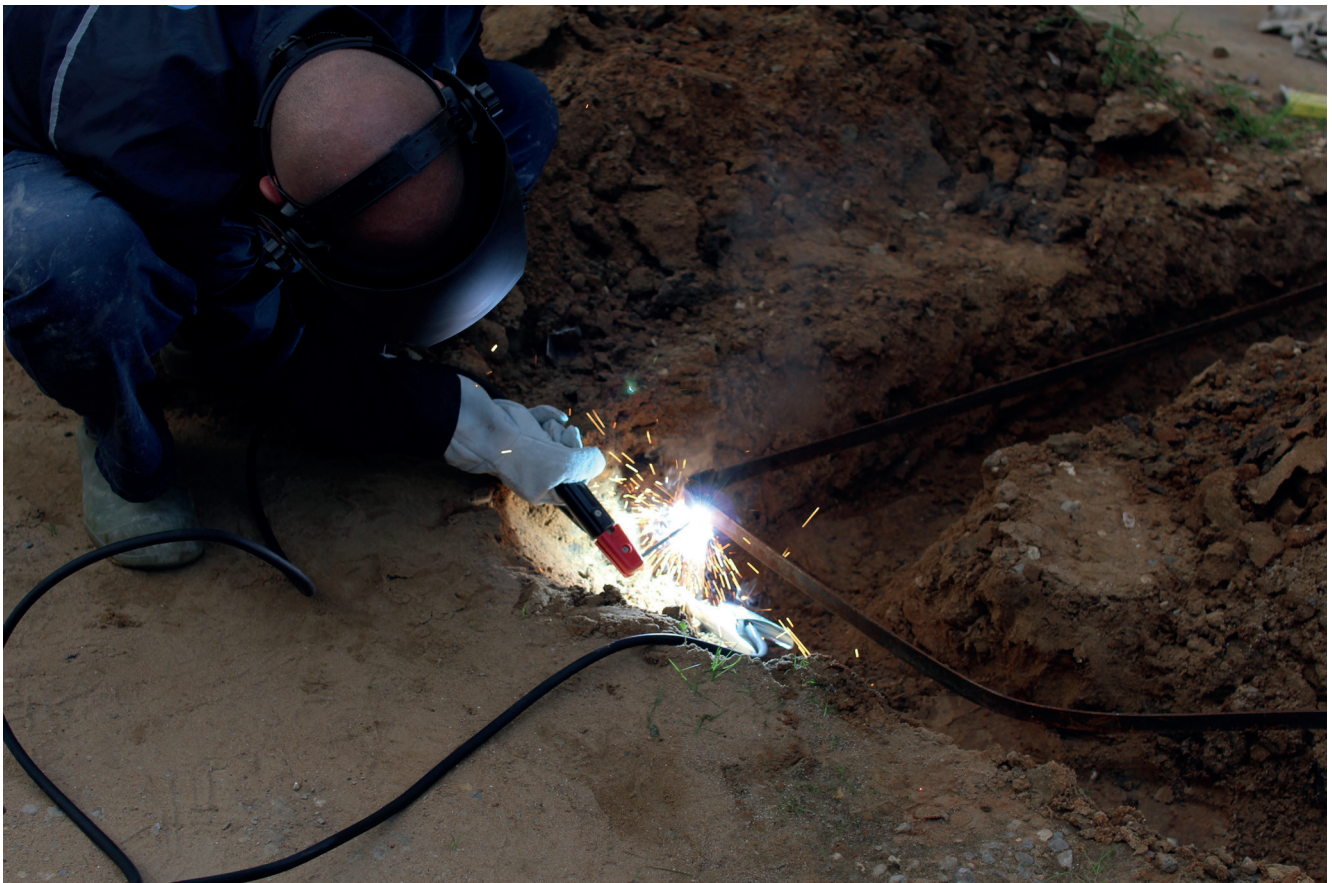
Example: Grounding / grounding pit
