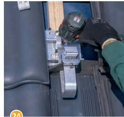
24 Fixate the position of the roof hook by tightening the bolt (6 Nm).
