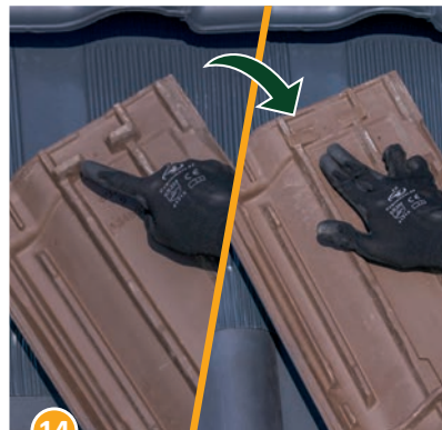
14 Remove the locking lugs from the back of the tiles that need to be put back in place.
