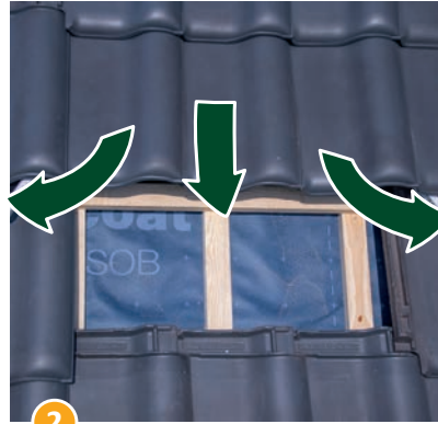
2 ...under the top row, so that the cross battening is easily visible and accessible.
